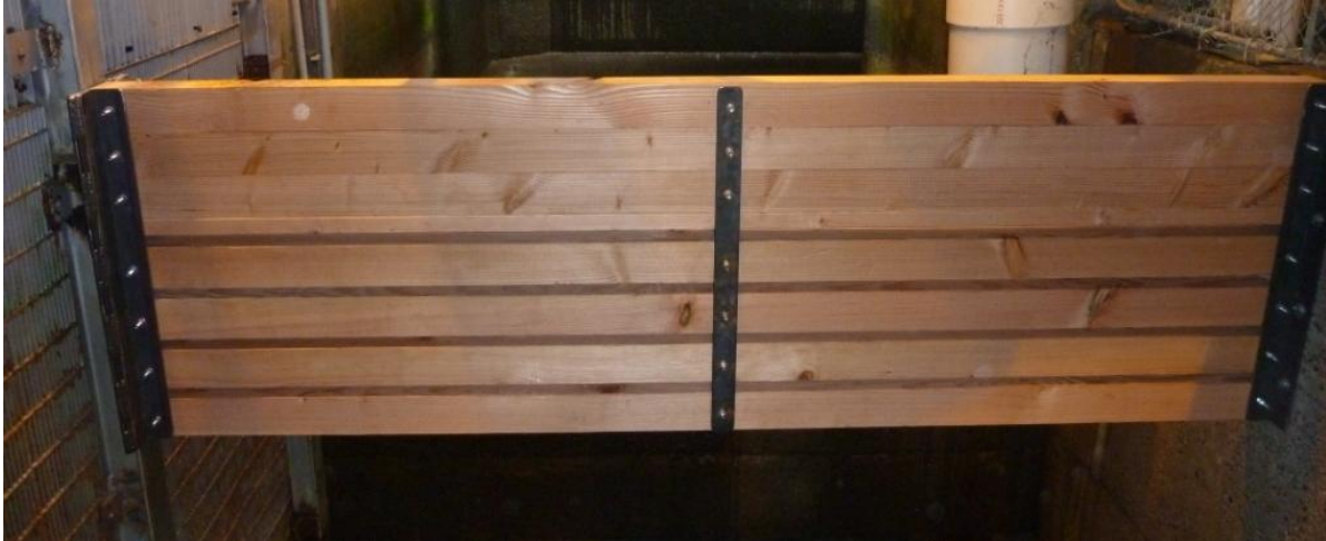
Figure 2: Baffle constructed in the AFF return pool looking upstream from the valve 15 trashrack.
