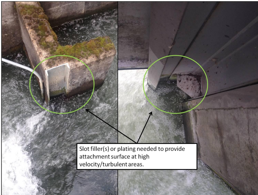
Figure 12 – Bulkhead guide slot (left) and irregular shaped frame (right).
