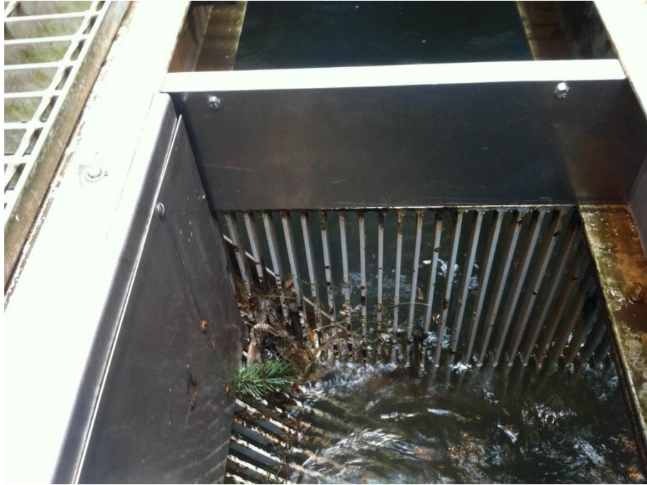
Figure 9: Improved raking transition from trashrack to walkway grating.
